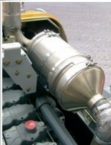
Diesel particle filter beneath cladding
