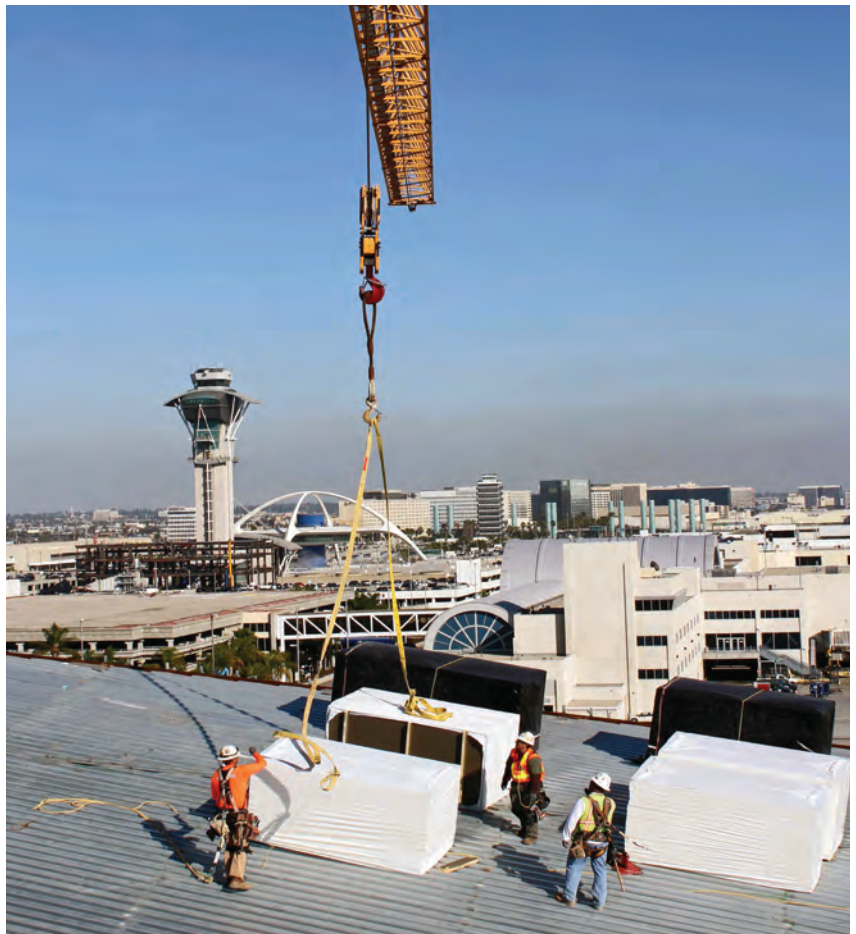
Upon completion in 2013, the Tom Bradley International Terminal will include one million square feet of space.
